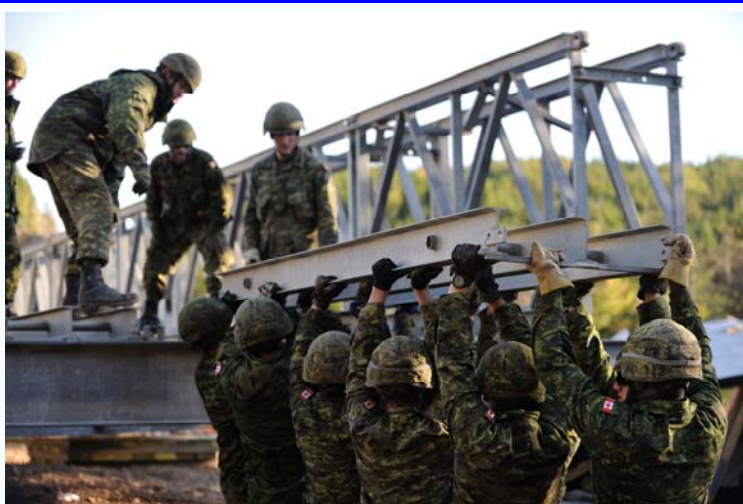
Engineers from 4 Engineer Support Regiment, in Gagetown, New Brunswick and 56 Engineer Squadron, in St. John's Newfoundland, lift a plain stringer into place during the construction of an ACROW Bridge in the small community of Trouty, after the main bridge was destroyed by Hurricane Igor.
